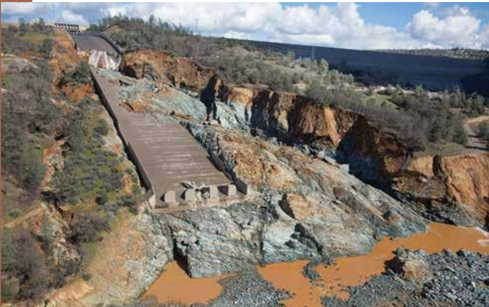
Oroville Dam Spillway, Feb. 27, 2017.
